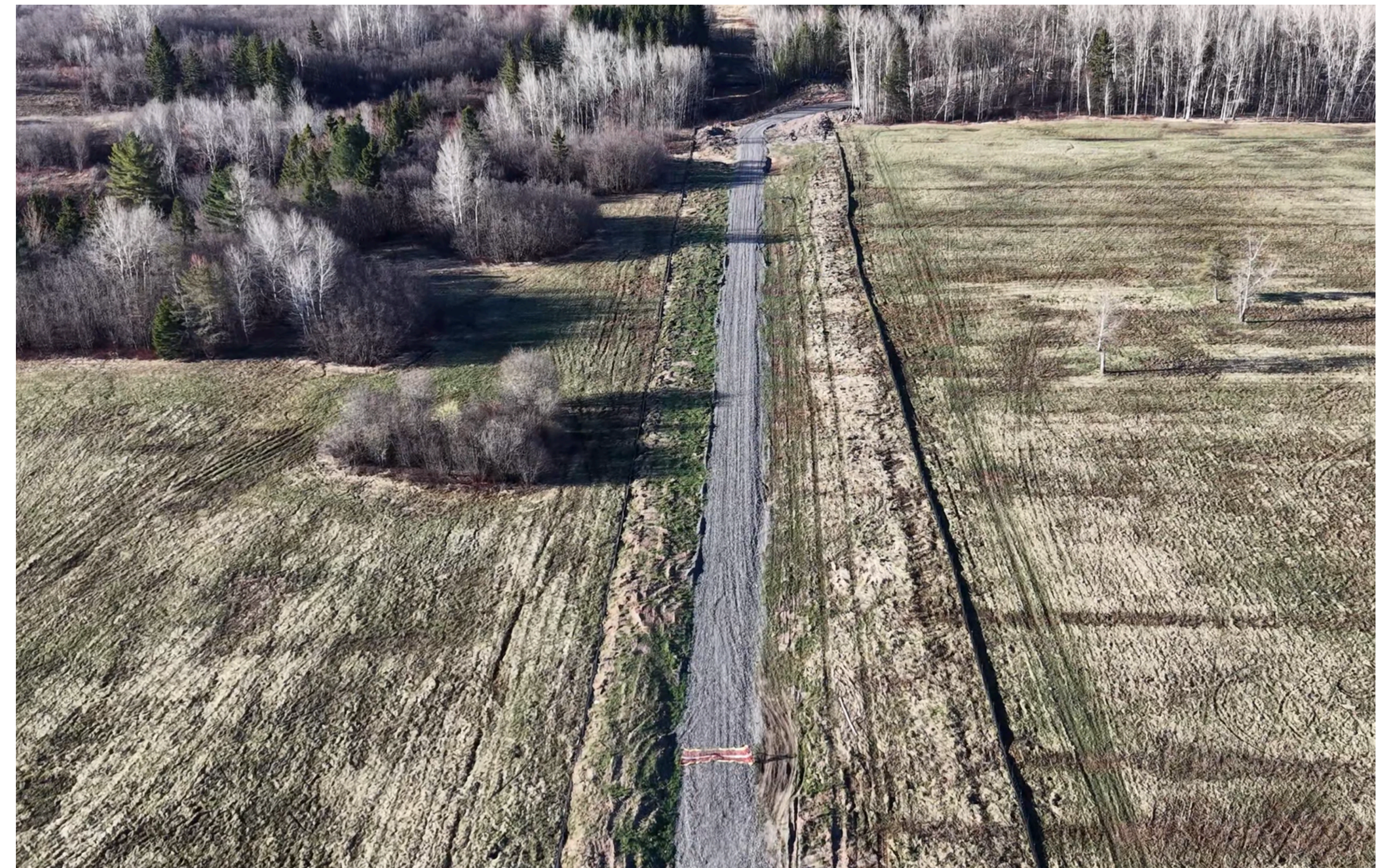
Vegetation clearing & Access Roads along Route (example shown near Third Line W)
